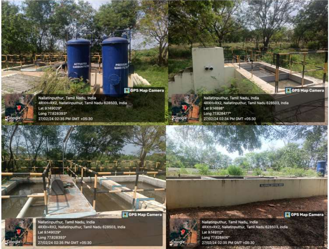
Photographic view of Sewage water treatment
